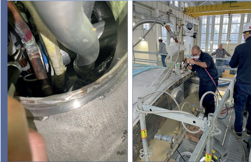
Localization and repair of the nitrogen loop of the solenoid thermal shield
