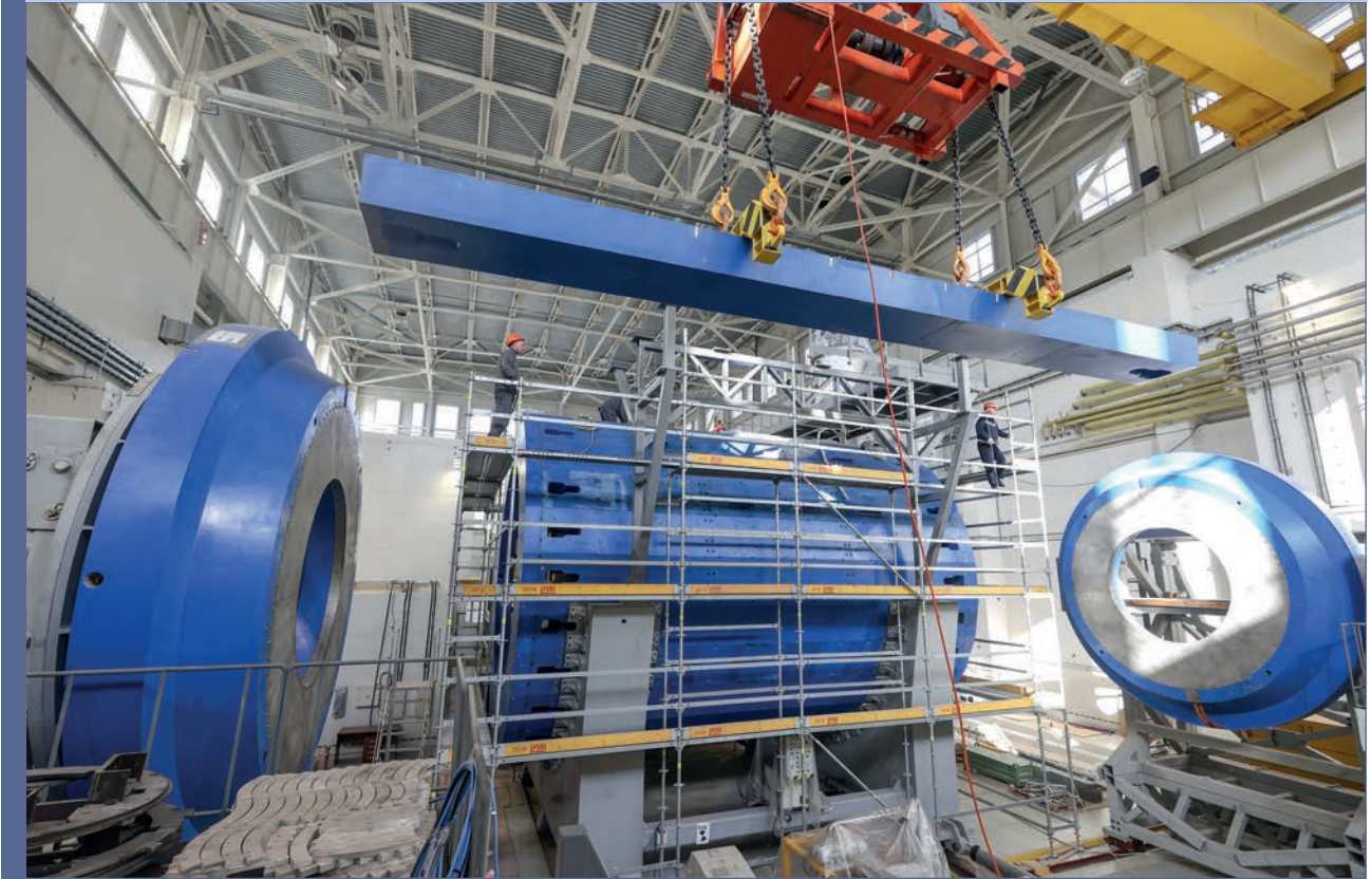
Installation of the last three beams of the magnetic core of the MPD detector
