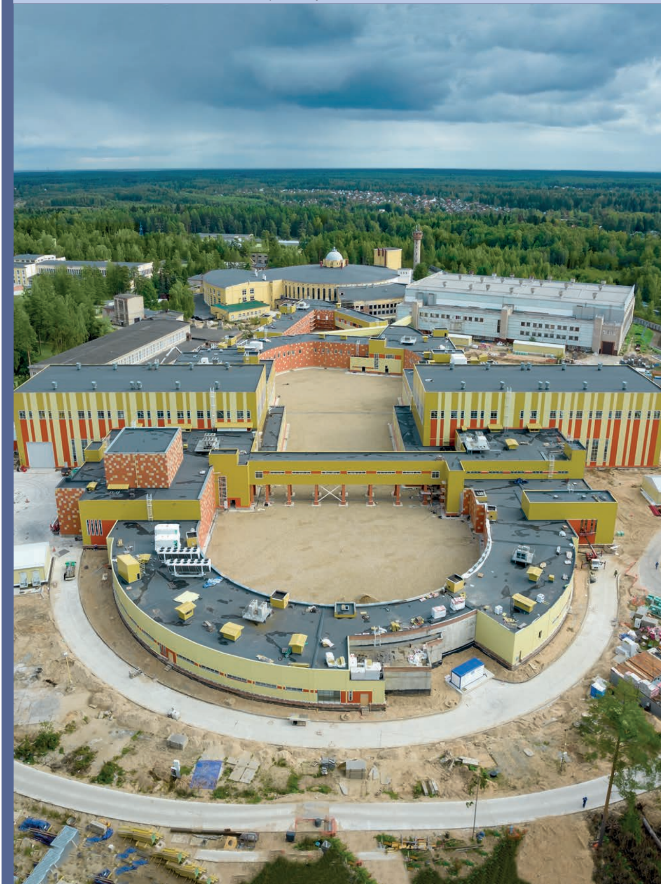
March. The construction site of the NICA collider. General construction works have been completed by 80%
