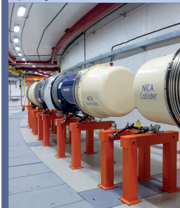
Dipole magnets installed inside the collider's tunnel
